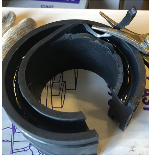
The rear installation will required cutting off the top inner ring to get a very tight fit and easier installation.
