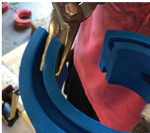
7. Due to the tight fit of the gap, top inner ring was cut off for easier installation process
